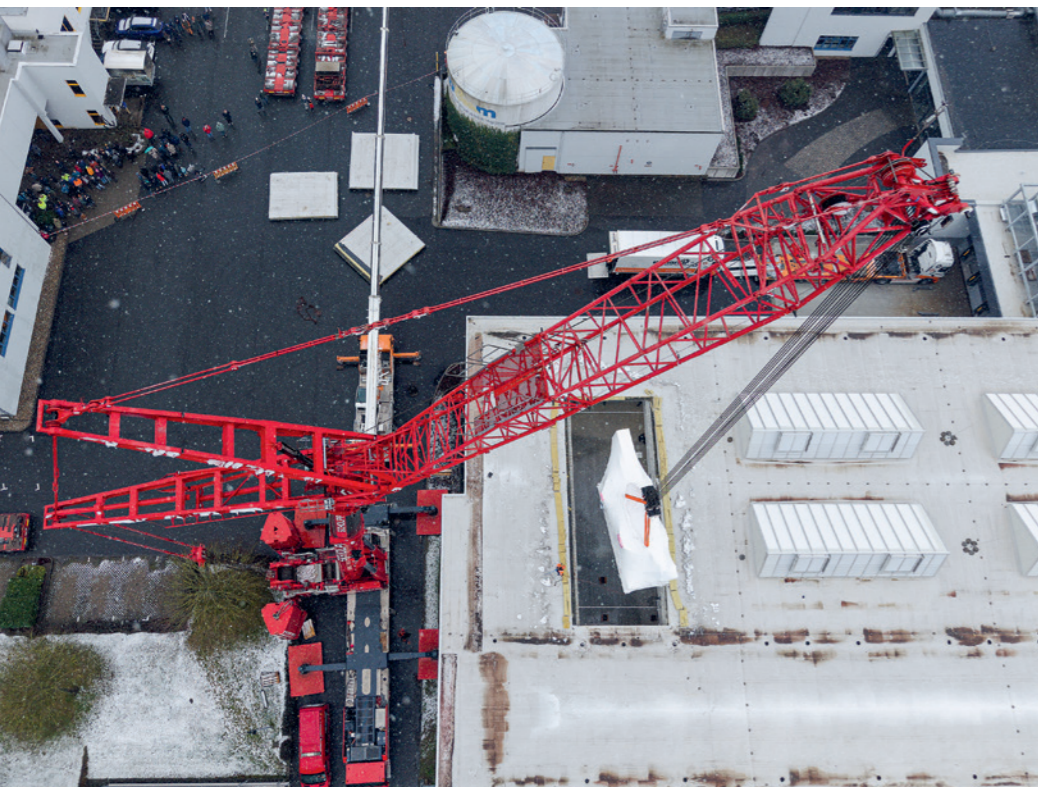
100 tons of steel as a special freight: The main body of the worldwide largest flat-die rolling machine is being lifted into the new Baier & Michels production site. © b&m
